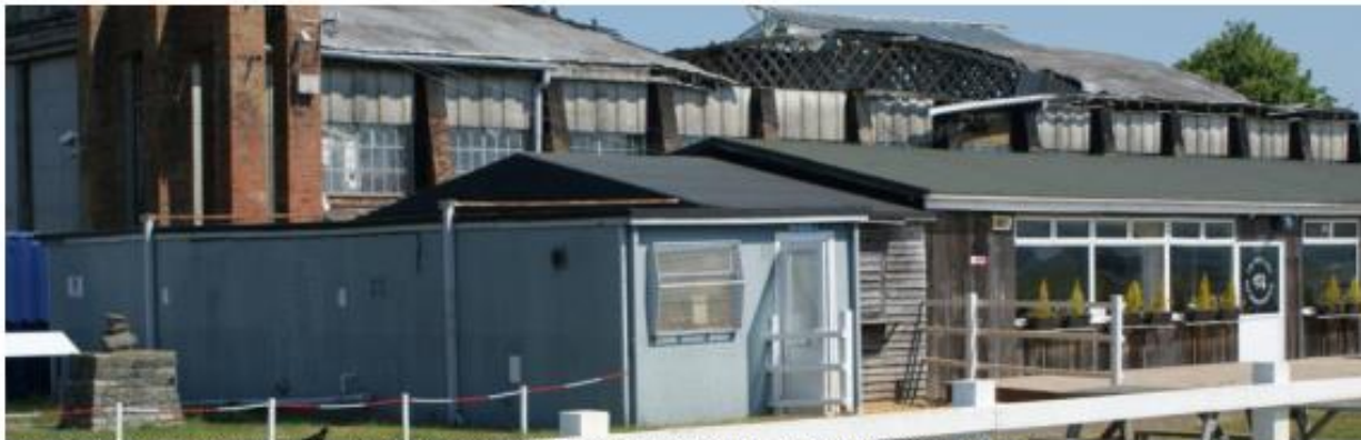
May 2023 View from the south - single story buildings are generally poor 1980. The former Flight Commanders office is to the right - see subsection 8 for fuller description of this building
