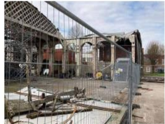
Worst area of collapse
