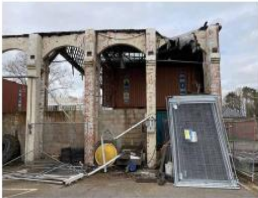
Central brick arcading with missing roof
